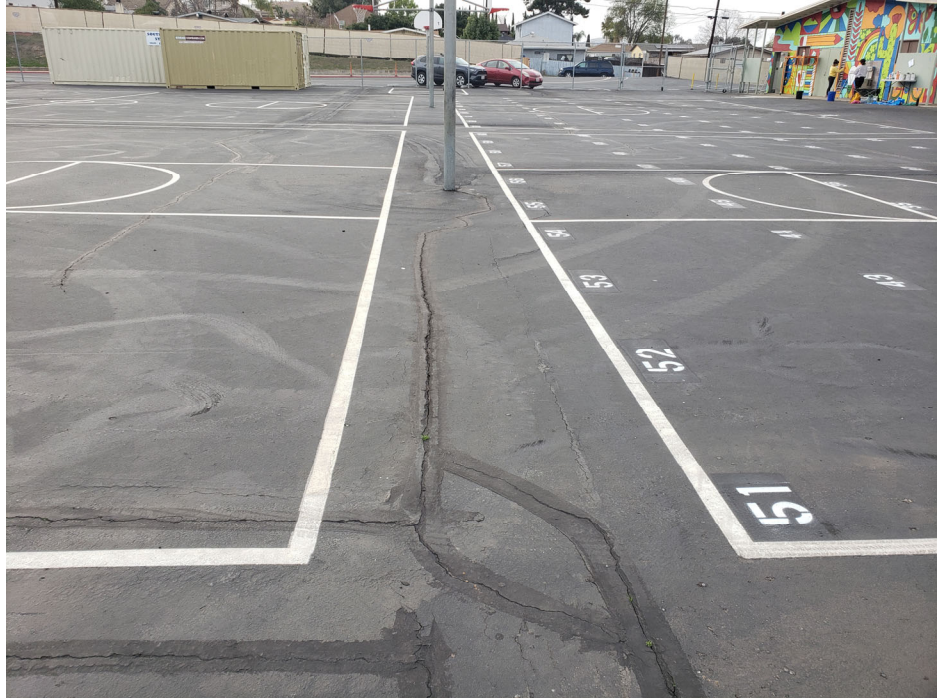
Photograph 7: West Hardcourt: View of play area looking west. Open cracks and previously patched cracks.
