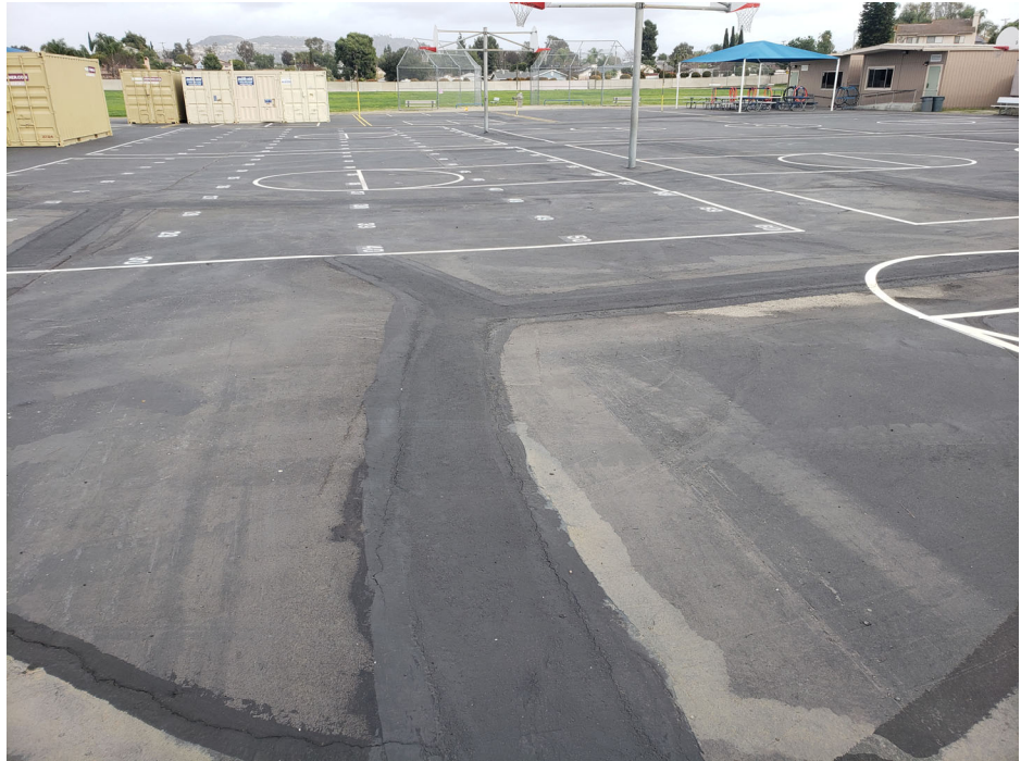
Photograph 5: West Hardcourt: Overall view of play area looking east. Open cracks and previously patched cracks.
