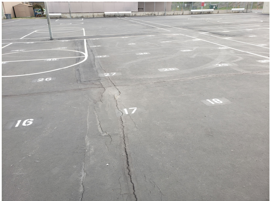
Photograph 8: West Hardcourt: View of play area looking south. Open cracks and previously patched cracks reopening.
