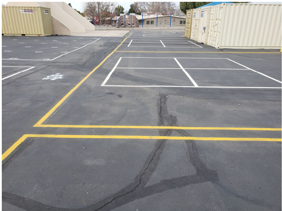
Photograph 6: West Hardcourt: View of play area looking north. Open cracks and previously patched cracks.
