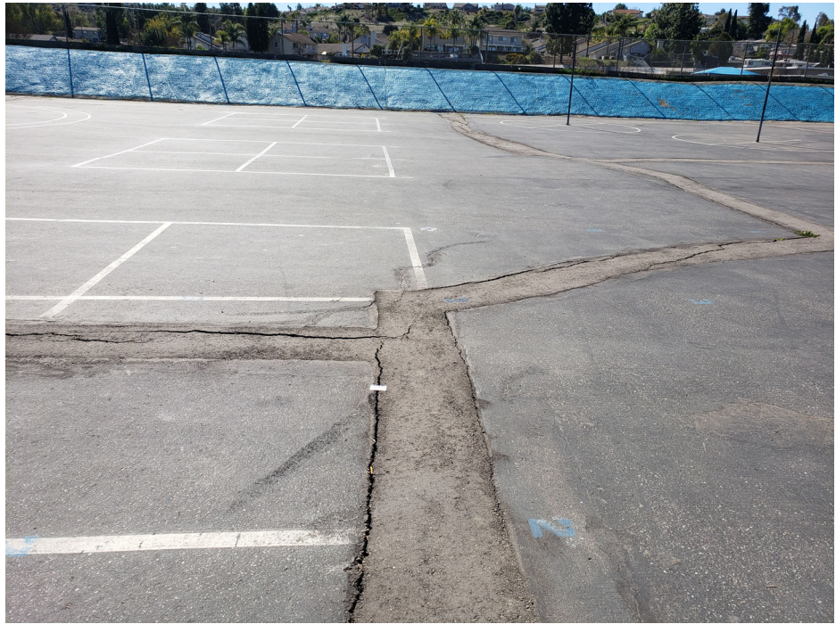
Photograph 3: North Hardcourt: View of play area looking south. Previously patched cracks reopening.
