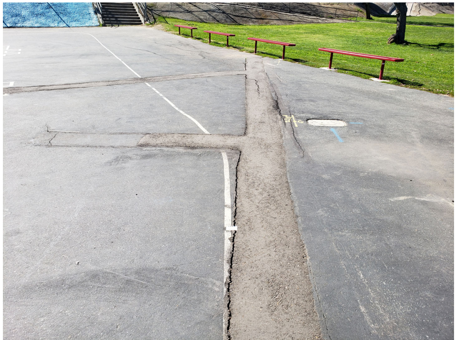
Photograph 4: North Hardcourt: View of play area looking west. Previously patched cracks reopening.
